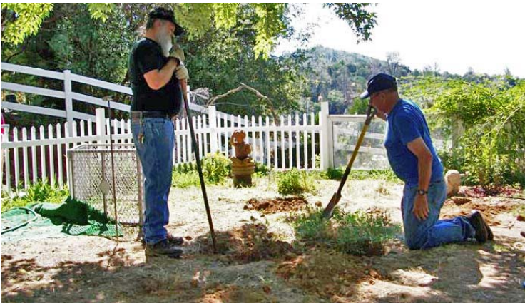
Charles Long & George Miskovsky search for lost septic tank with detectors, shovels & knees
